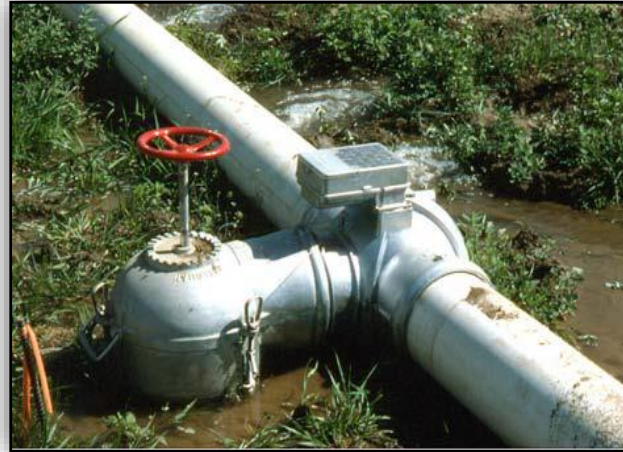
Improved Gated Pipe
